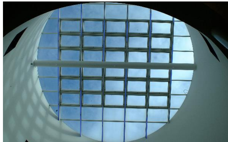
Casement Roof Vents
